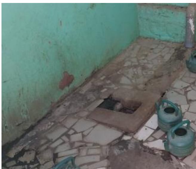
Photo 10 CS Khasso Latrines mal entretenue
