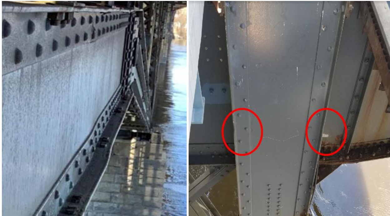
Figure 10-13: Deformation due to buckling
