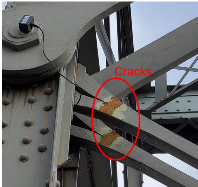
Figure 10-16: Cracks in the eye-bars
