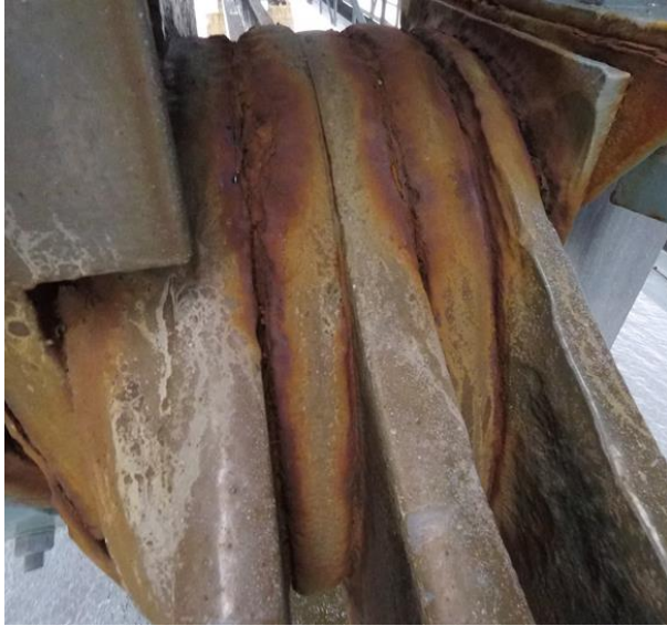
Figure 10-14: Eye-bar assembly showing corrosion
