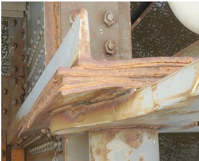
Figure 10-15: Rust jacking – the build up of corrosion material between members
