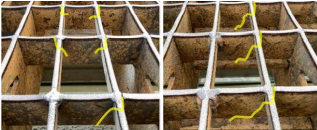
Figure 10-5: Cracks in East lane grating that require repair
