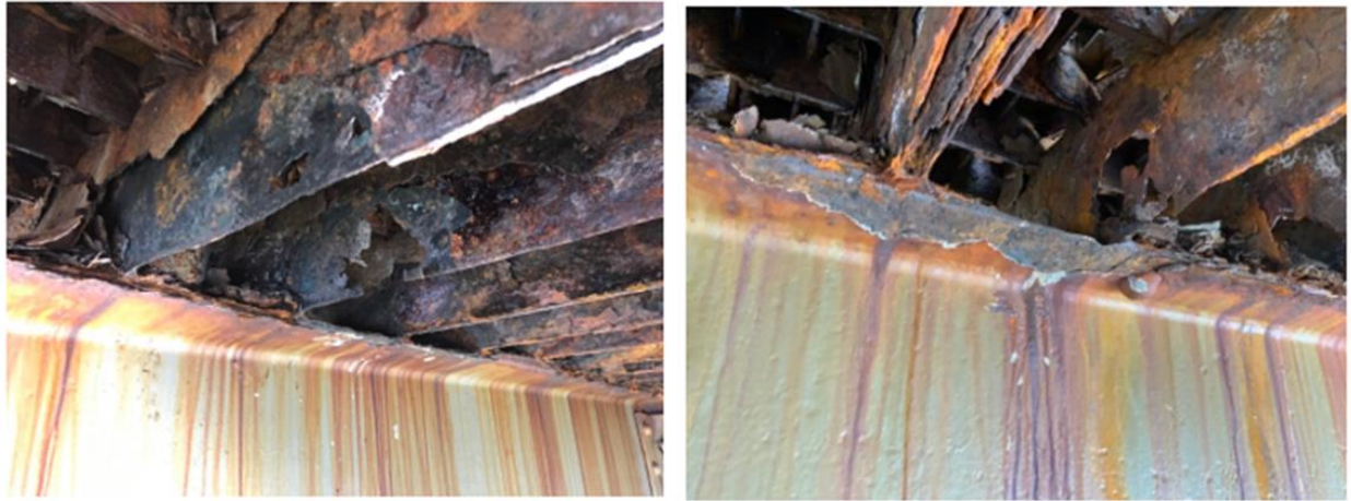
Figure 10-3: Condition of the grating under the Boardwalk
