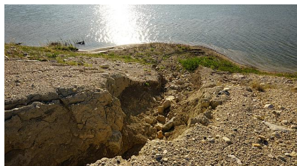
F: Gully in Channel Side-Slope and Sediment Accumulation (mini-delta)
