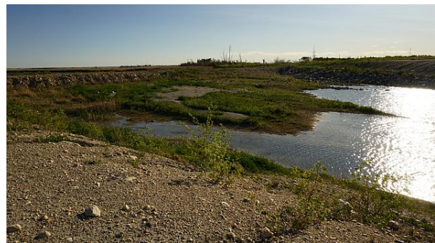
D: Sedimentation on the Channel Side of the Cut-off Berm
