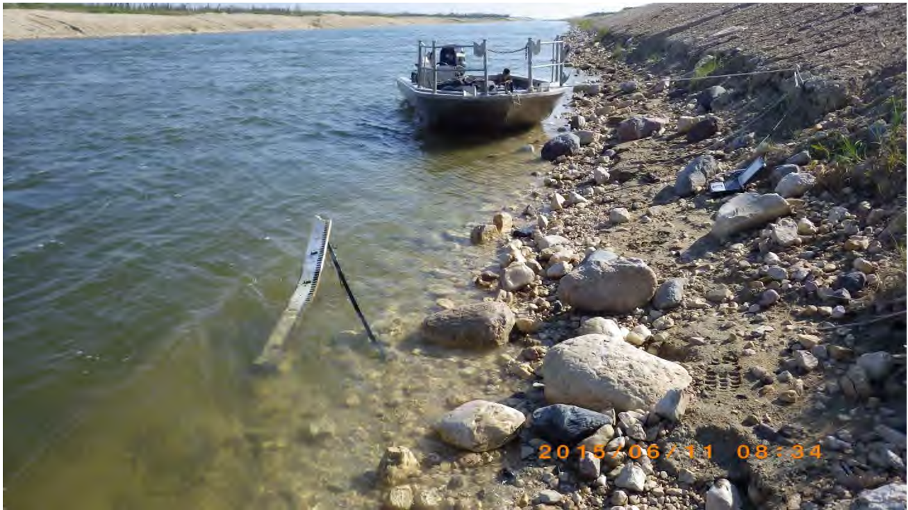
Photo 1. Damaged Gaugeboard at Reach 1 Bench Mark R1-I-A, looking east D/S
