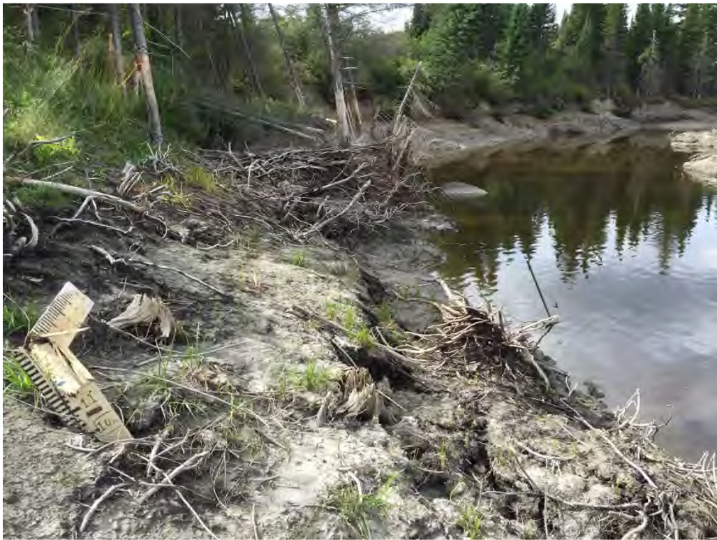
Photo 5: Damaged gauge board and slope failure, looking D/S from BC-TM.
