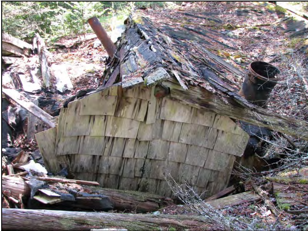
PLATE 8: Site 1: Remains of collapsed wooden structure; facing southwest.
