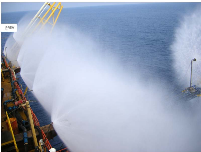
Photo 2 Rigside Cooling System (Source: Optima 2014)
