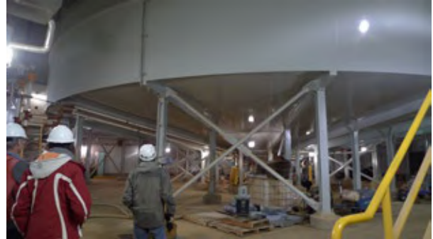
Exhibit 9: The water treatment facility at Equity Silver Mine in central B.C.
