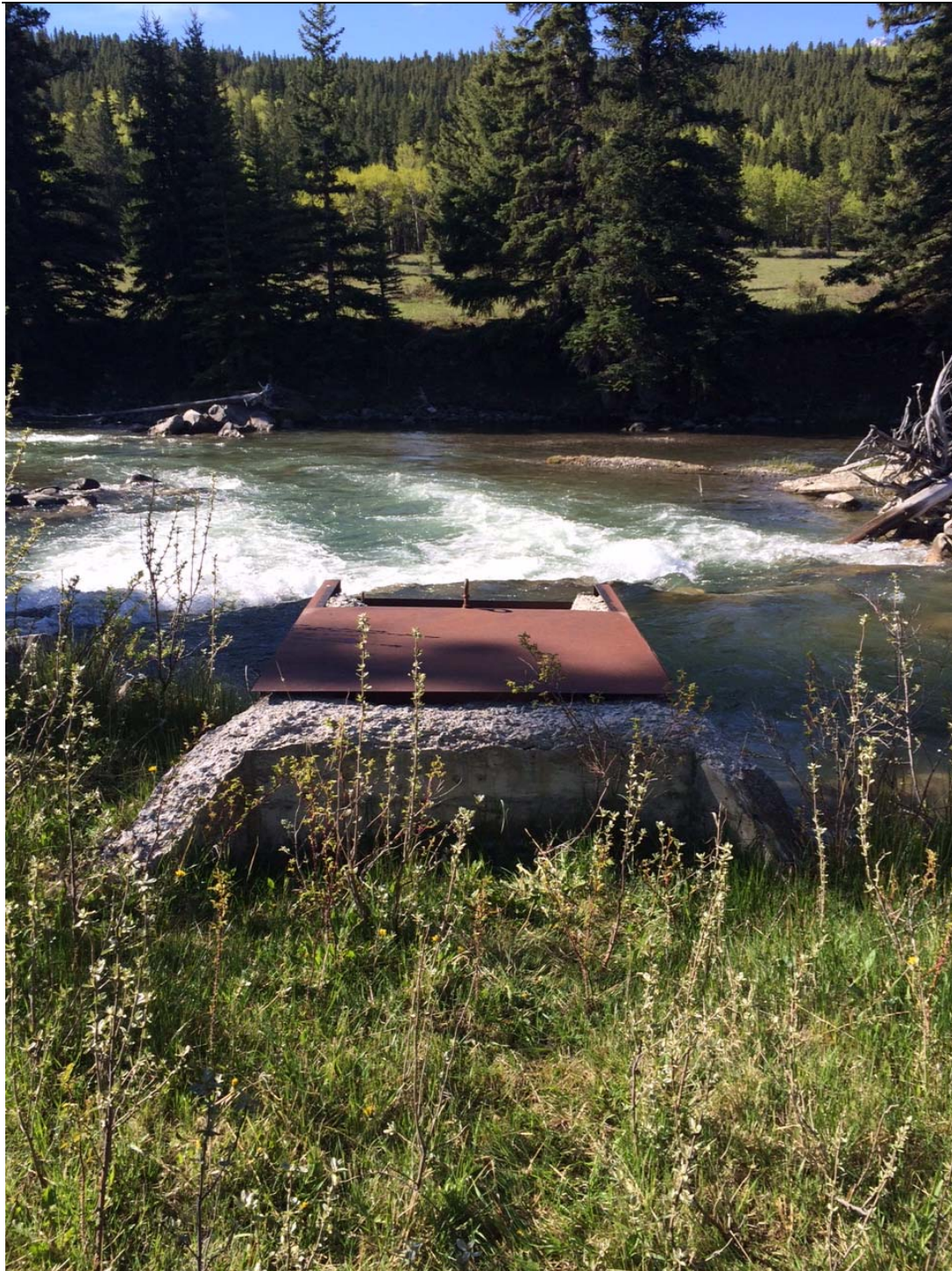
Photo 1 – Devon Water Intake on the Crowsnest River
