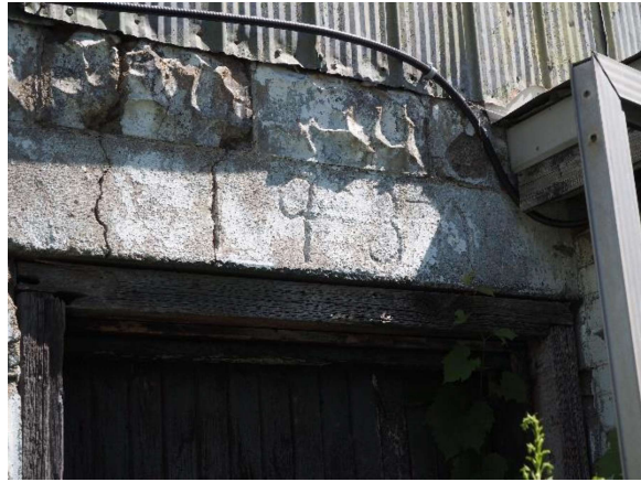
Plate 42: Cracked lintel above south entrance door
