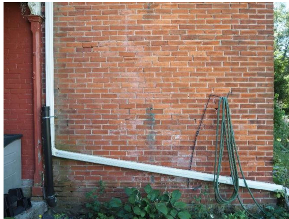
Plate 38: Efflorescence and missing mortar on west elevation near entrance porch
