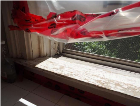
Plate 33: Work paint on windowsill of second floor bathroom, front unit
