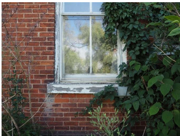
Plate 39: Worn paint on trim surrounding windows
