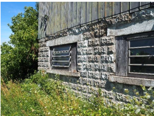
Plate 22: Rusticated concrete foundation, windows, and metal cladding on south façade, looking northwest
