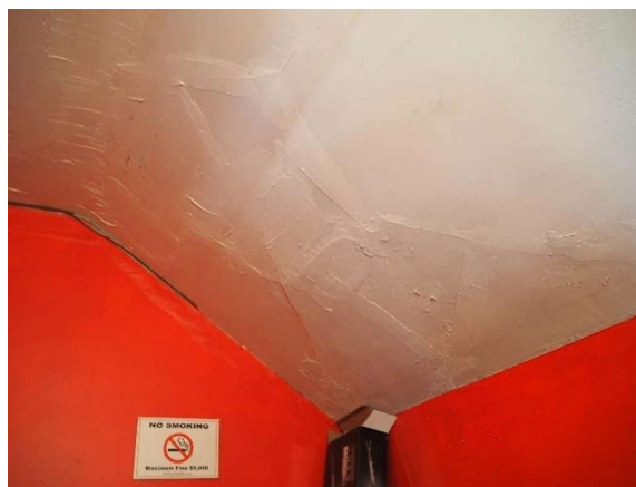
Plate 32: Patched cracked plaster on second floor bedroom of front unit
