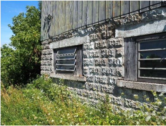
Plate 41: Rusticated concrete block foundation with limited cracking
