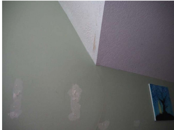
Plate 34: Patched plaster cracks in second floor laundry room of rear unit
