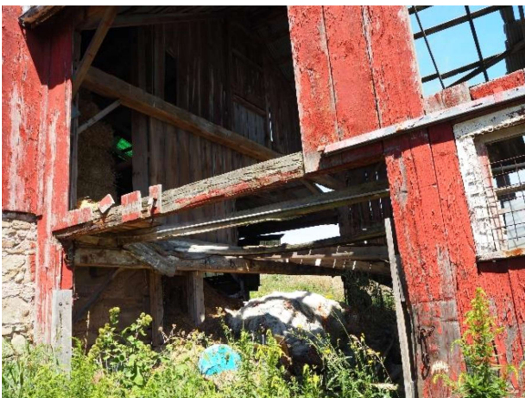
Plate 27: View of partially collapsed roof and hand hewn beams
