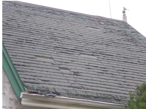
Plate 31: Roofing in poor condition
