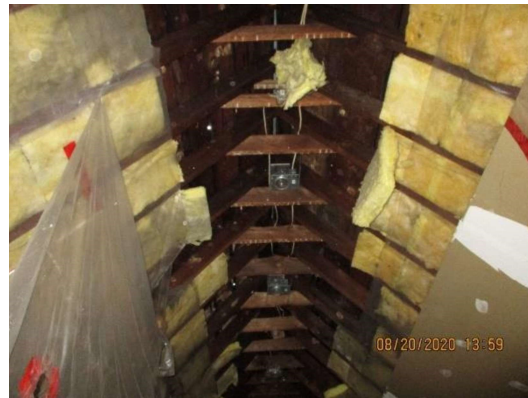
Plate 35: Water damage from roof leak
