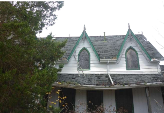
Plate 32: Sagging east porch
