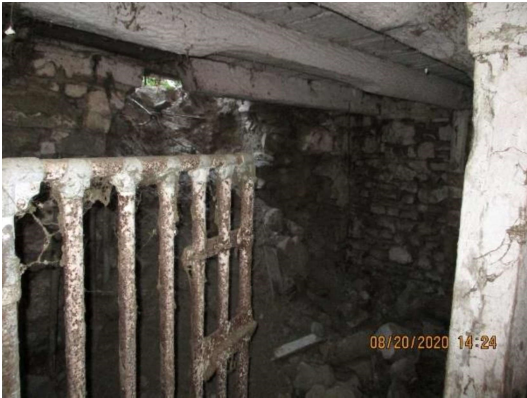
Plate 38: Gap in foundation
