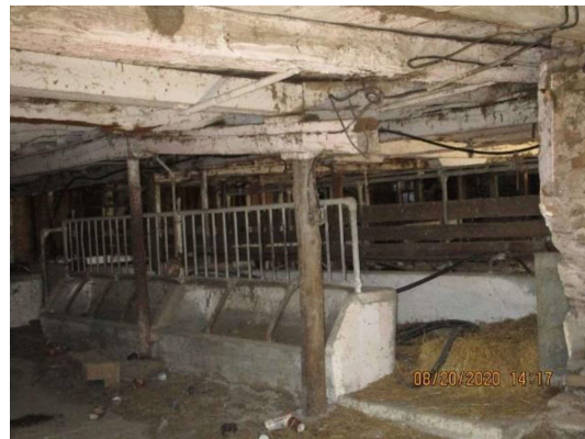
Plate 41: Interior structural beam of questionable integrity
