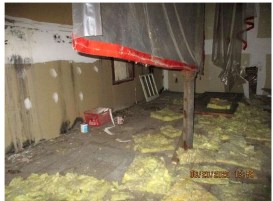
Plate 33: Water damaged drywall and black mould
