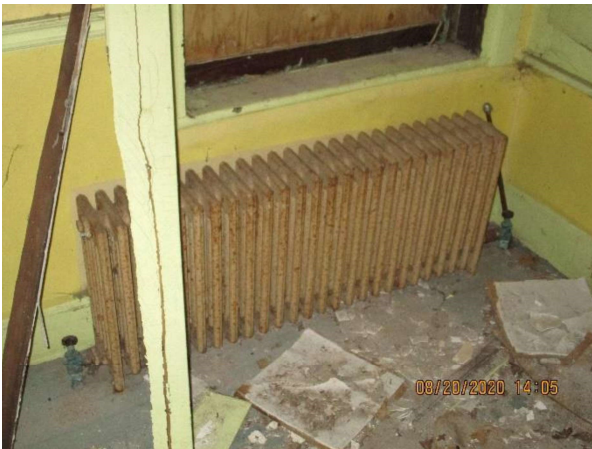
Plate 14: Interior main floor radiator and debris
