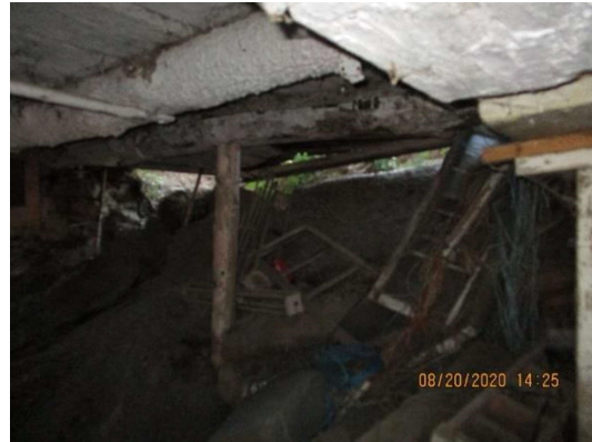
Plate 39: Collapsed foundation wall
