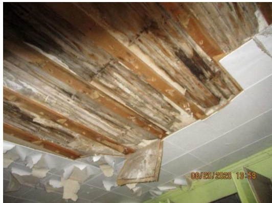
Plate 34: Water damaged ceiling tiles
