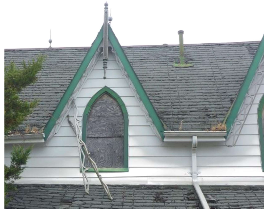
Plate 29: Worn paint and damaged bargeboard
