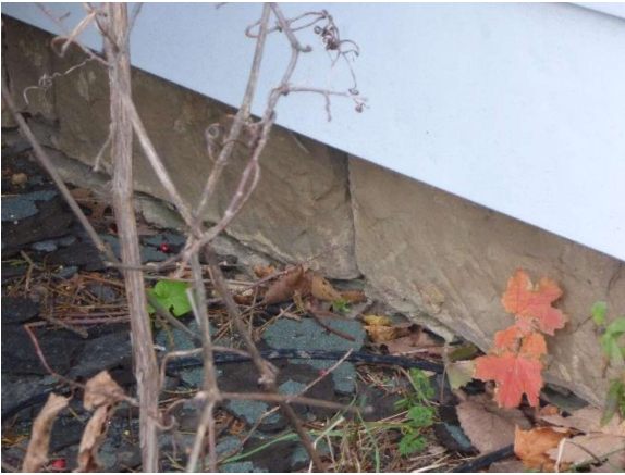
Plate 28: Detail of foundation gaps
