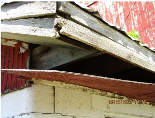
Plate 40: Collapsing exterior structural beams
