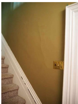
Plate 16: Localized plaster cracks in the entrance hallway
