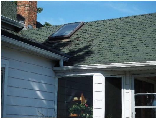
Plate 12: Localized areas of lifting shingles
