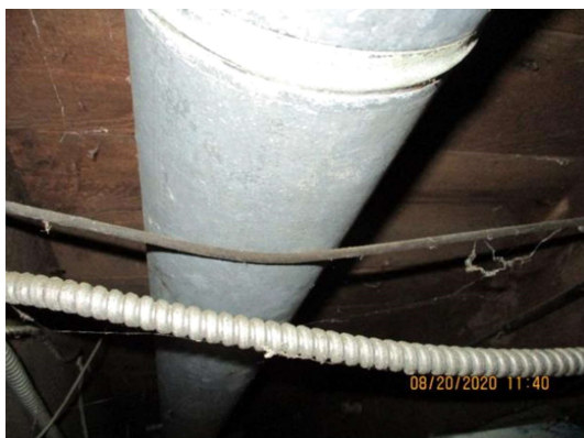
Plate 20: Knob and Tube wiring without protect from a forced air duct
