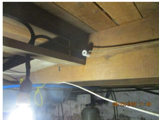
Plate 19: Active Knob and Tube wiring feeding light
