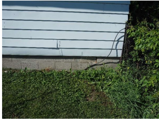
Plate 13: Settling and refilled cracks in the addition's foundation
