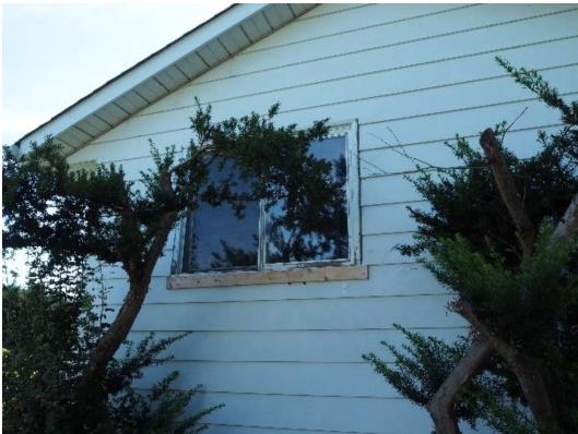
Plate 14: Northwest window with evidence of water intrusion
