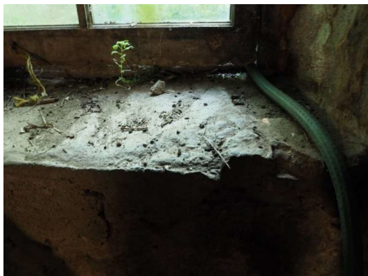
Plate 18: Gaps around basement windows
