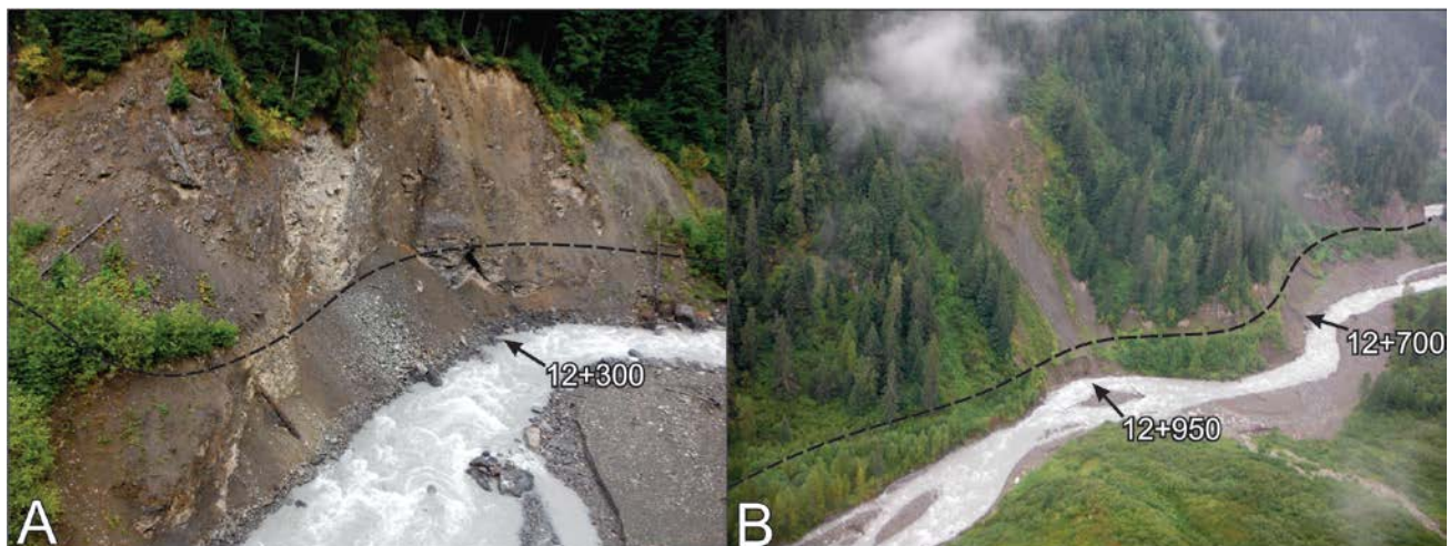
Figure 6-3: Recent lateral erosion at A) Station 12+300; and B) 12+700 and 12+950. Black arrows denote direction of channel migration; dashed line shows approximate proposed access road route.
