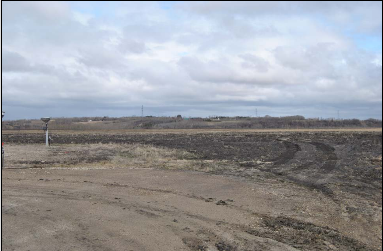
Photograph 6: A view facing west of the on-site expansion area for the rail yard that has had topsoil salvaged (May 6, 2014).
