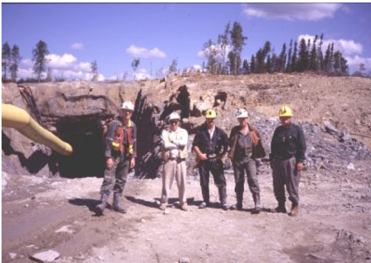
Figure 6-1. Portal/decline access to the Thunder Lake Deposit Main Zone gold mineralization for bulk sampling; 1998 Teck Cominco and Corona Gold joint venture (MNDM, 1998).
