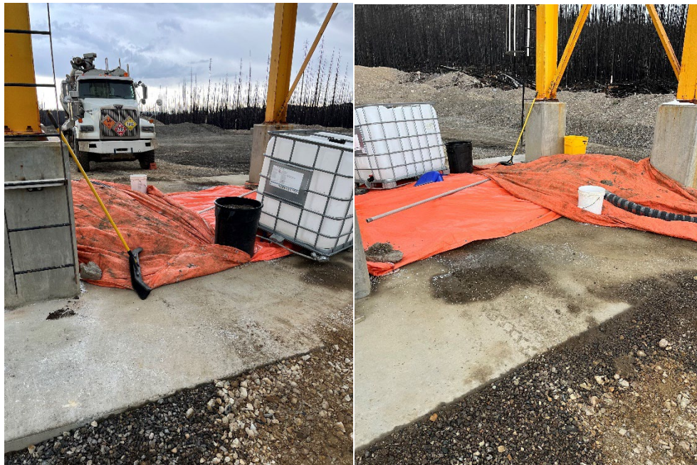
Photos 2 & 3: Spill Cleanup In Progress
