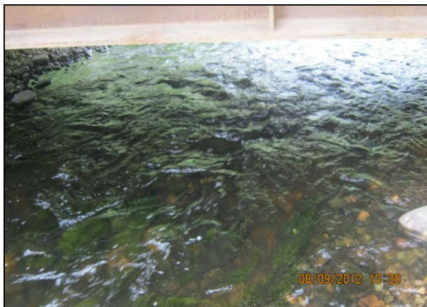
Plate 35. Mine Access Road crossing AP-007 Turtle Creek, bridge and shallow bars, September 9, 2012
