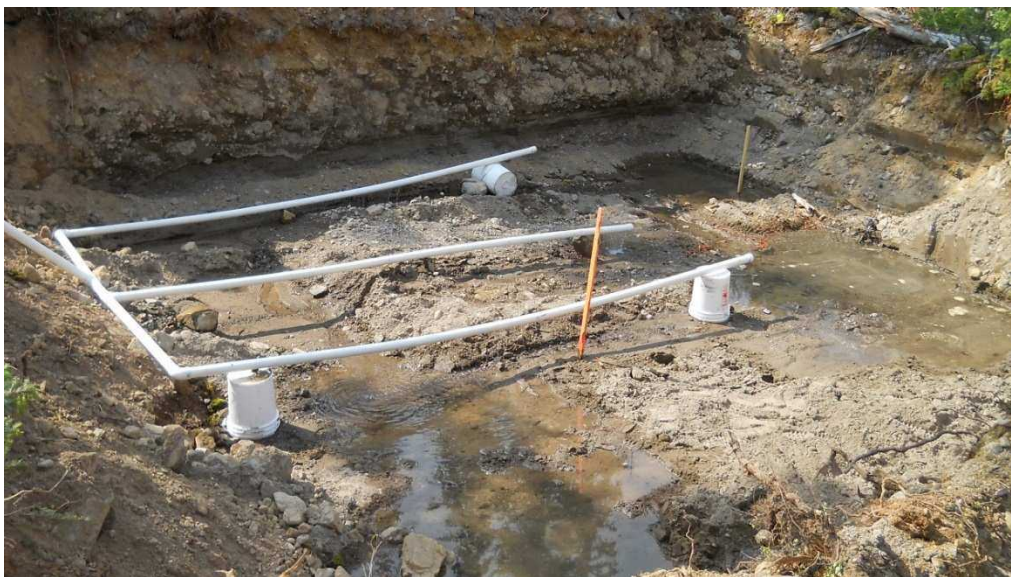
Photo 2: RIB Pilot Loading Test after two days of loading at 93 m 3 /day (17 US gpm), July 19, 2013.
