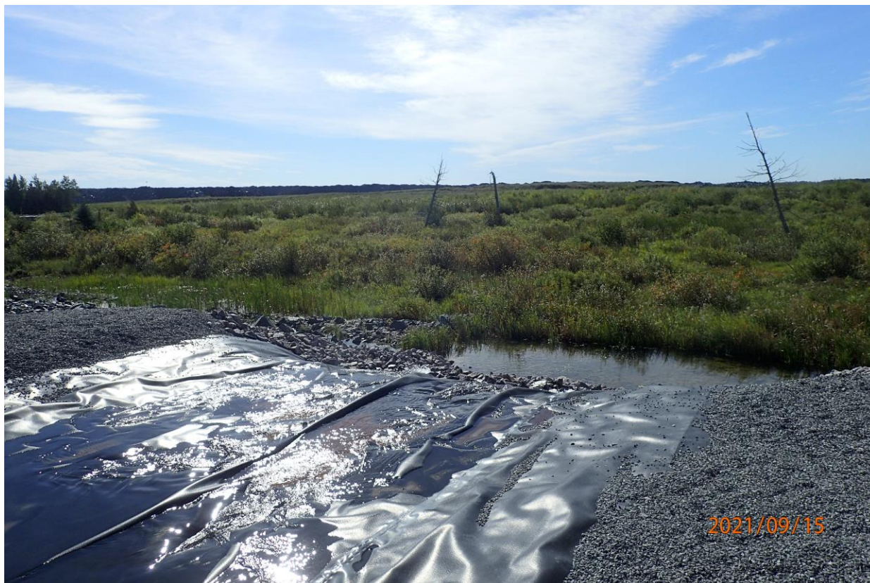
Photo 1: Outflow Basin emergency spillway active.
