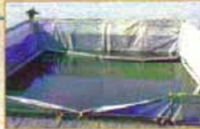
Example of Silt Curtain
