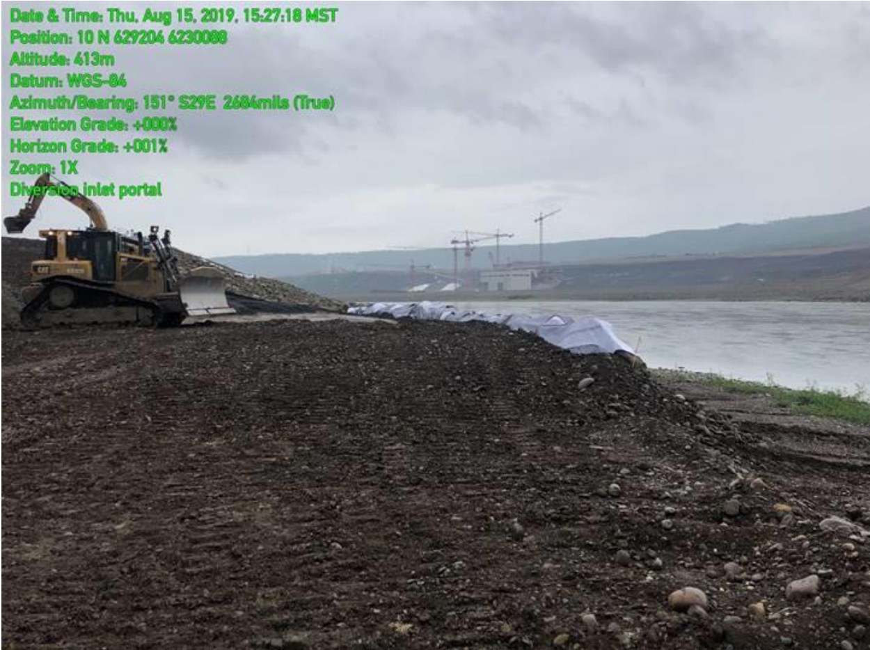
Figure 6. Debris and sediment are prevented from entering the Peace River at RSEM L5 (looking east) using rip rap and liner with mesh armouring (August 15, 2019).
