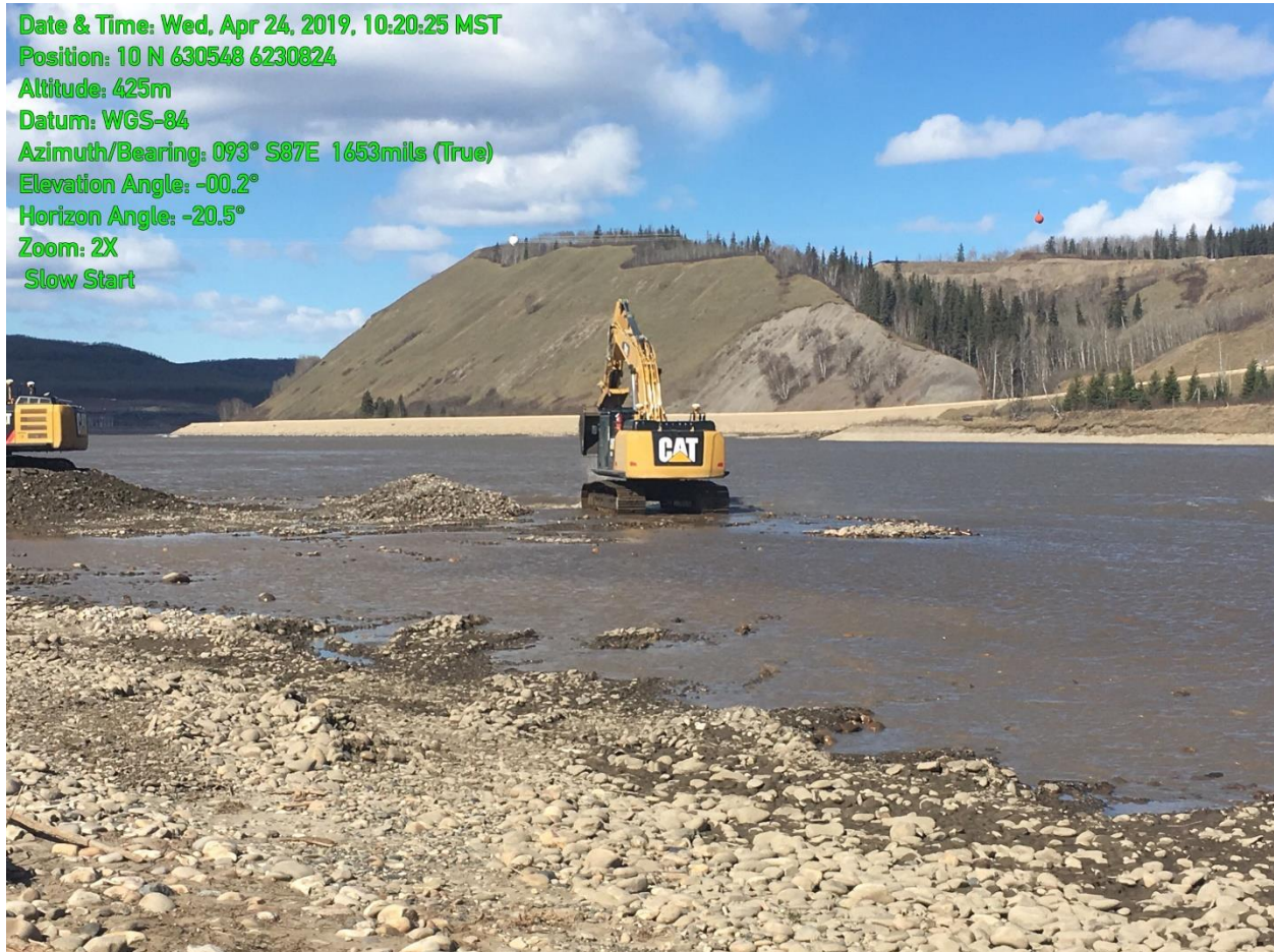
Figure 4. An excavator works to contour a bar in the Peace River at Site 108R to reduce potential for fish stranding. The excavator works in a slow, controlled and continuous manner to scare and exclude fish from the work area (April 24, 2019).
