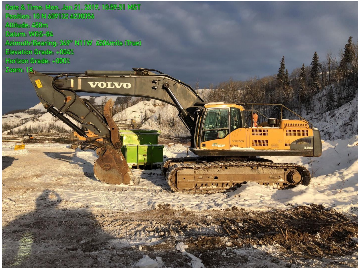
Figure 3. An excavator uses biodegradable hydraulic oil at Cache Creek during reservoir clearing activities (January 21, 2019).
