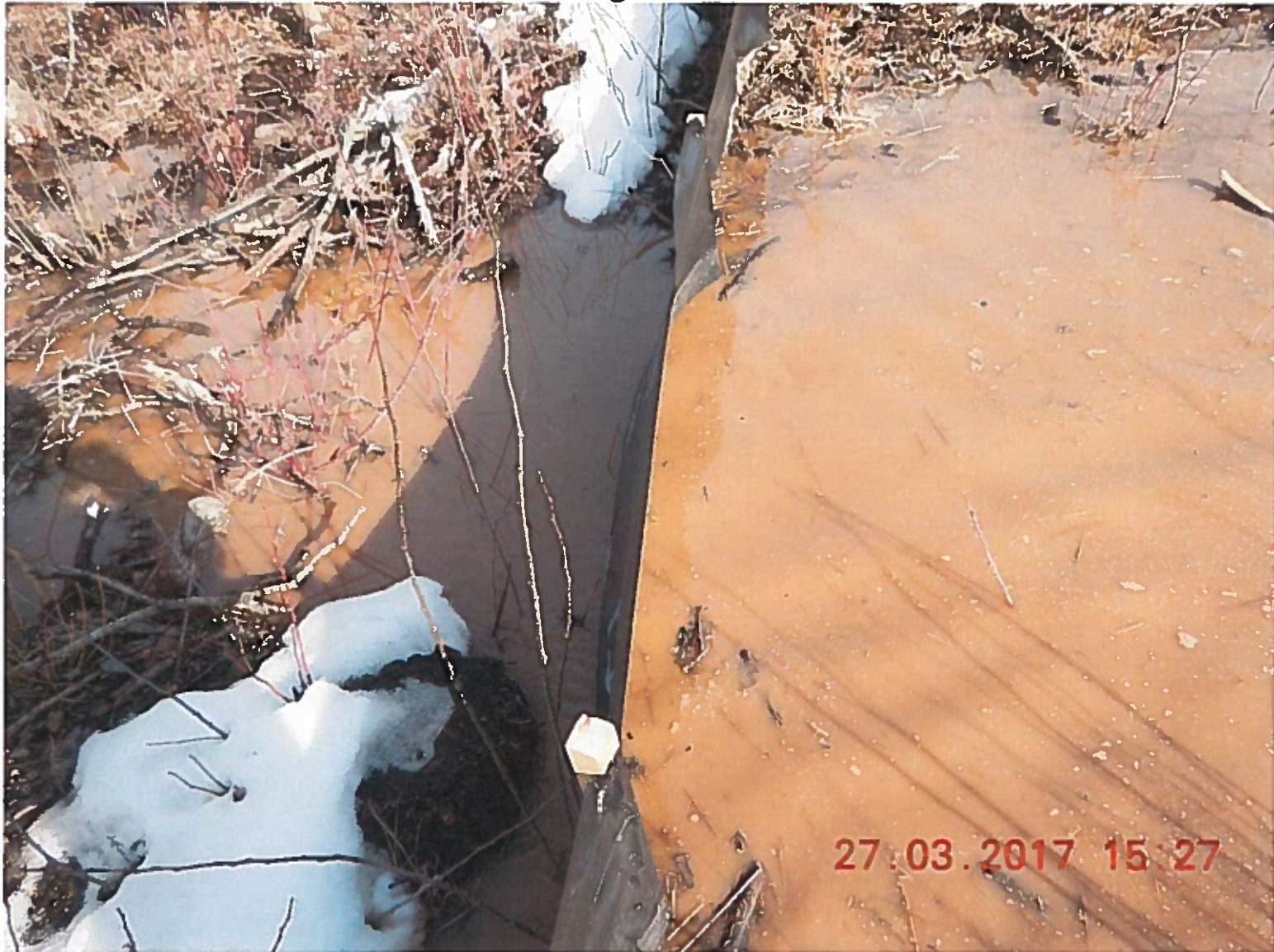
Figure 8: Sediment Laden water leaving Area A work area
