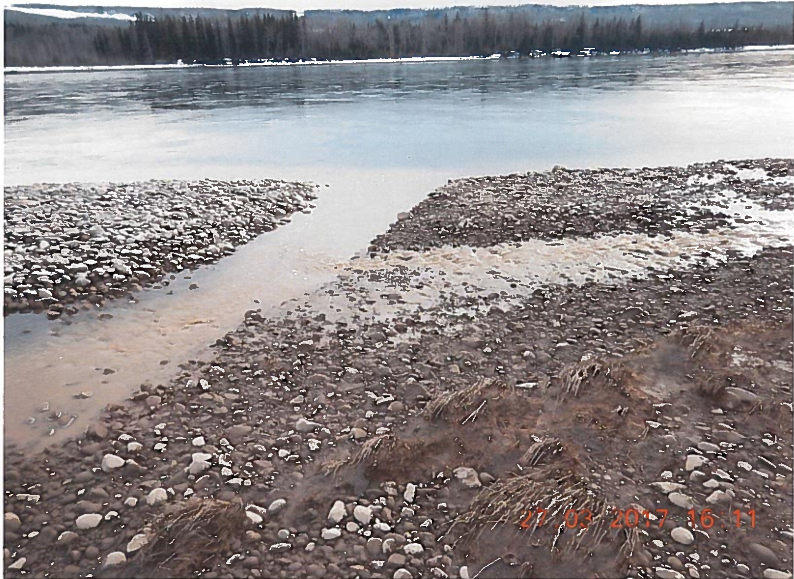
Figure 4: Sediment laden water exiting Unnamed Creek 3 culvert and entering the Peace River
