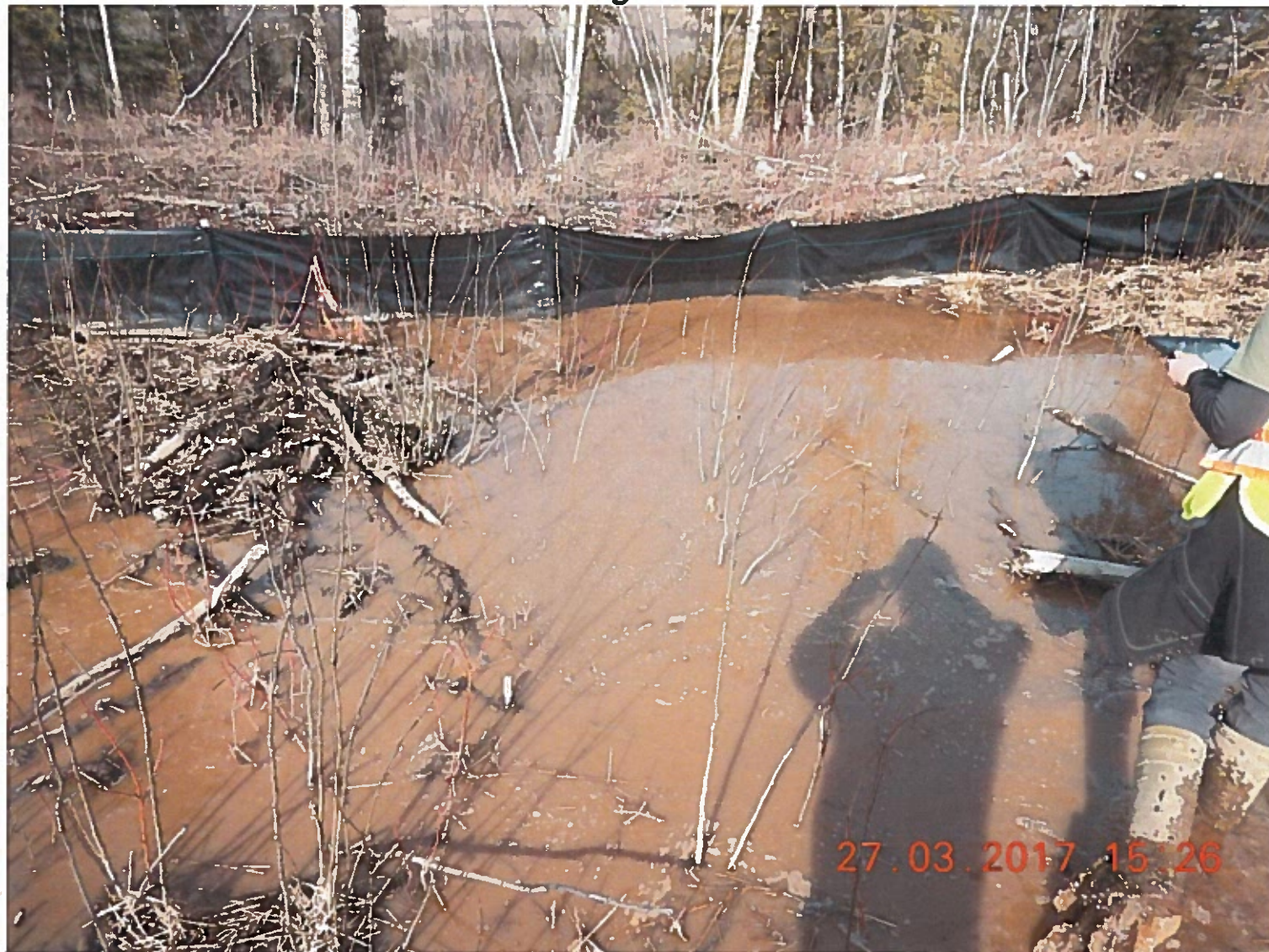
Figure 7: Sediment Laden water leaving Area A work area
