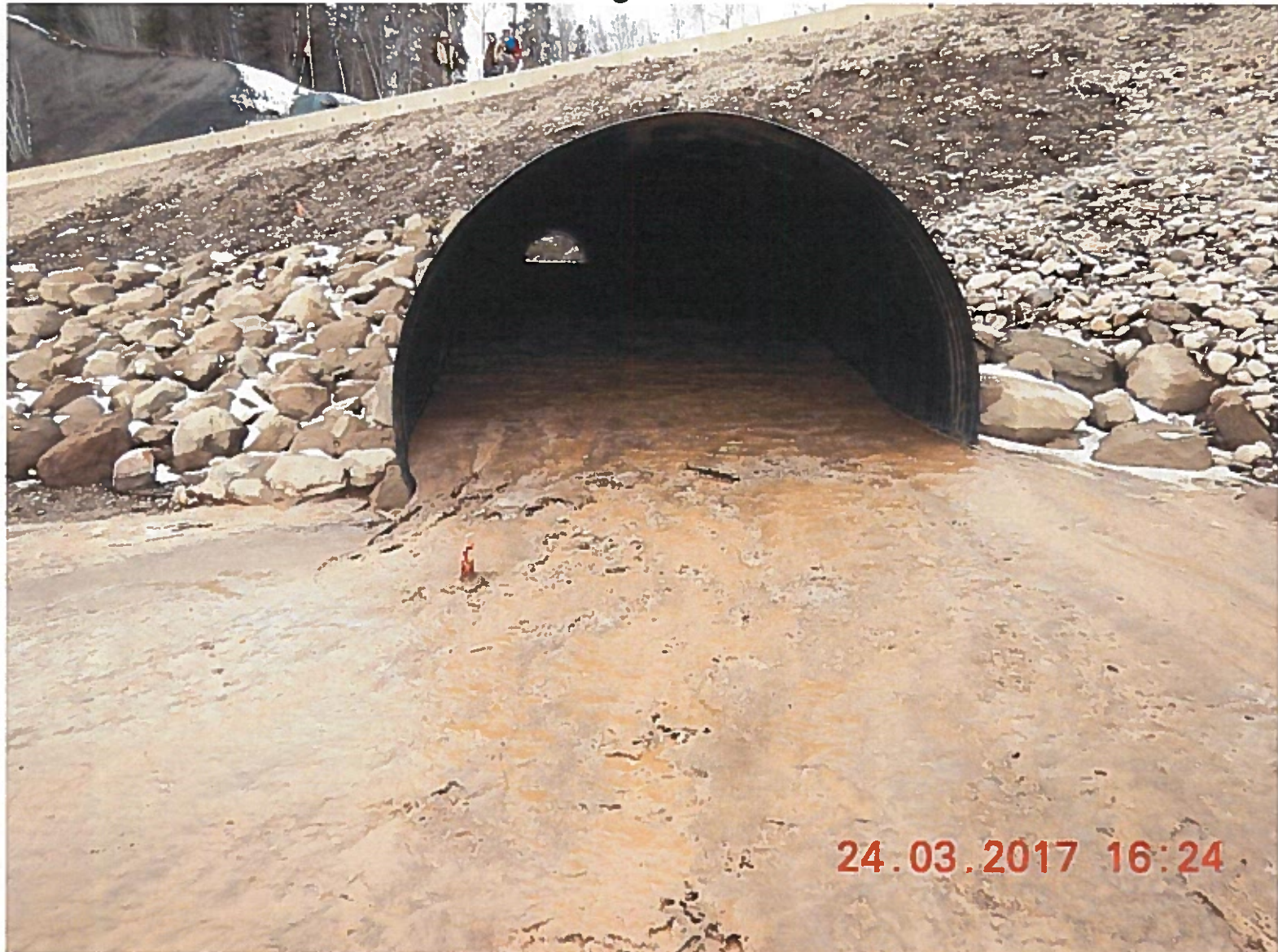
Figure 5: Sediment Laden water flowing through culvert under River Road
