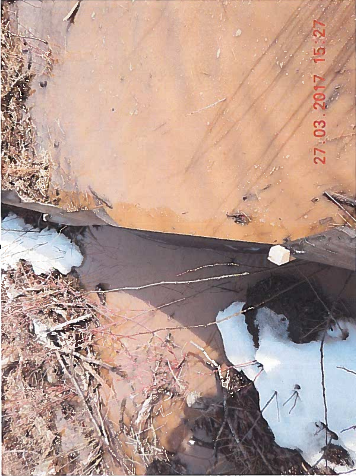
Figure 8: Sediment Laden water leaving Area A work area
