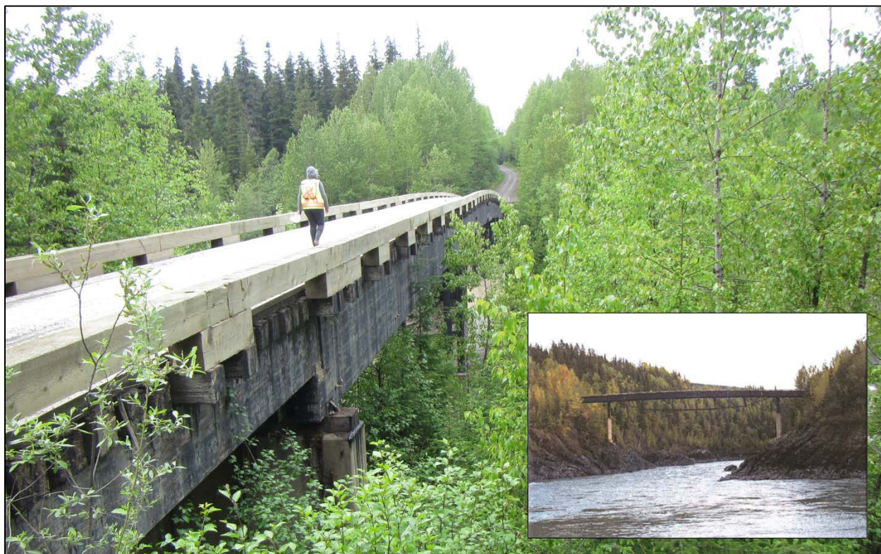
Figure 2-1 Photo of Nass River Bridge, facing east (inset: facing south) (photo: Avanti).
