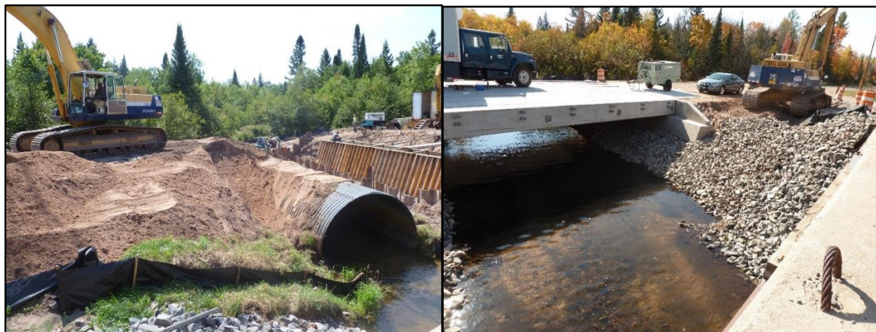
Left: Falls River culvert on Golf Course Road, Baraga County, Michigan, before removal. Right: Falls River Golf Course Road after culvert removal. Credit: E. Johnston, Keweenaw Bay Indian Community.
