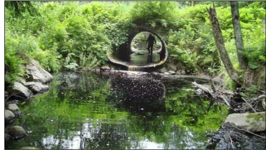
A culvert barrier. Credit: M. Fedora, U.S. Forest Service.
