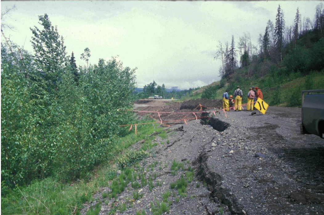
Figure 7: A reactivated slump earth flow after an up-grade of the Morice Road. Attempts to stabilize the road have cost millions of dollars over the past 30 years.
