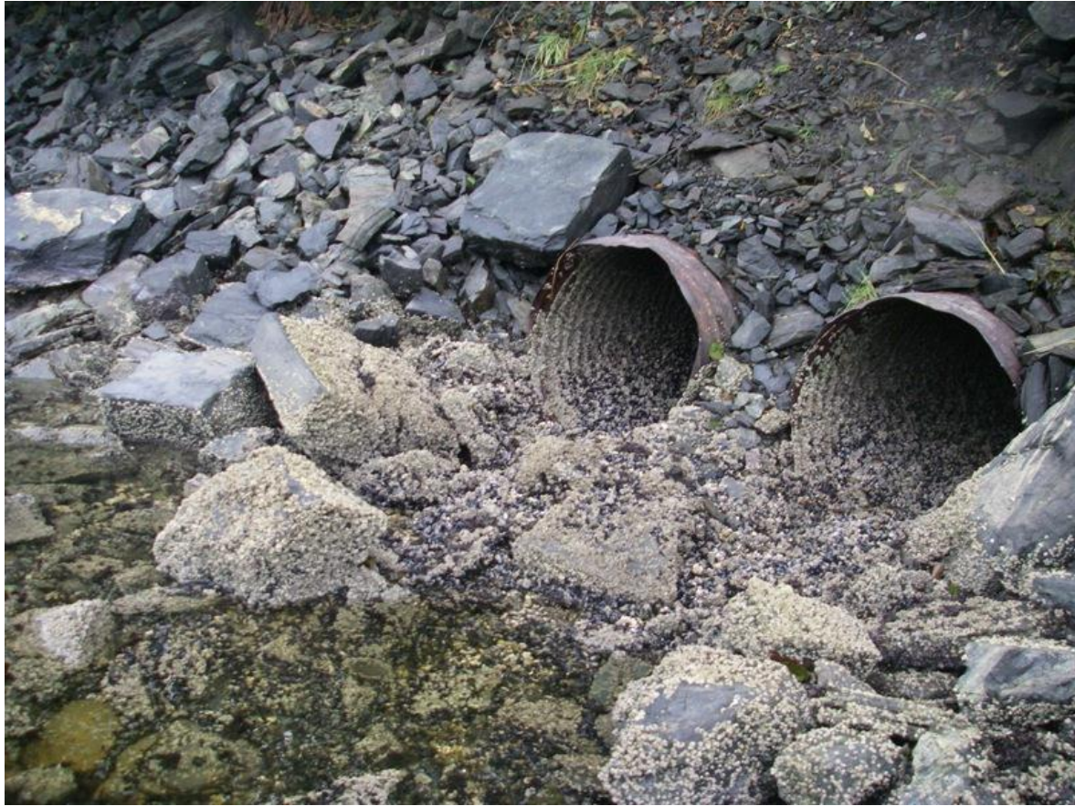
Photo 5: Two corrugated culverts on the pond side of the road. No connectivity occurs when tide levels are below the culverts.
