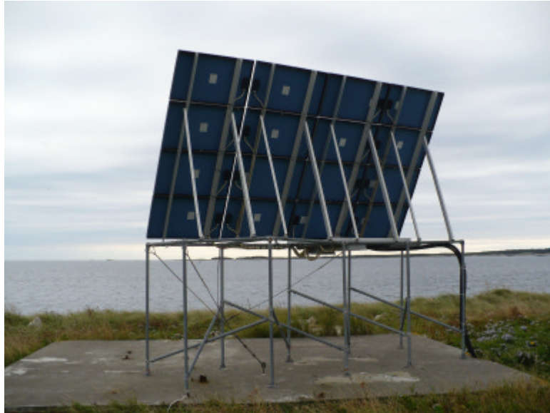
Figure 1e: Solar panels mounted on a concrete slab.
